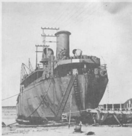
At its permanent berth on the beach at Anchorage, Alaska, the after end of the S.S. SACKETT'S HARBOR supplements the city's power system with a 5400-kw. marine turbine-electric plant.
